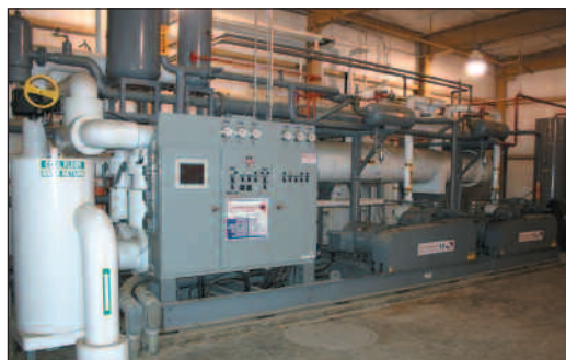
Vilter 450 XL reciprocating refrigeration compressors provide the durability and performance to maintain the Pavilion's ice sheet at exactly the right temperature, 24/7, month after month.
