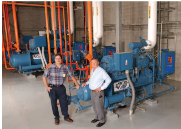
Ice Plant Refrigeration Supervisor Richard Cogburn (left) selected six Vilter compressors to eliminate noise and vibration-related maintenance issues. Source: Vilter Manufacturing.
